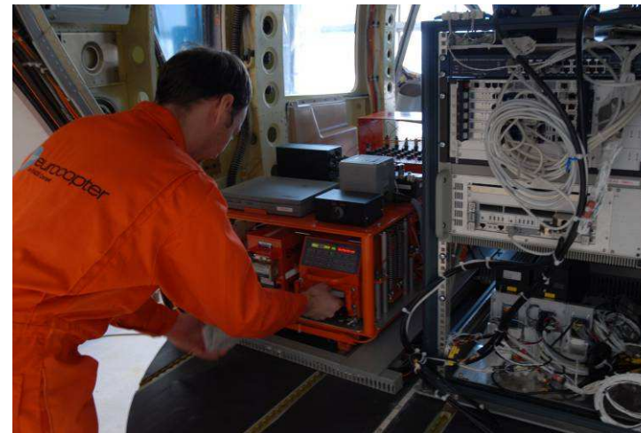
SATCOM equipment in a rack (right)
